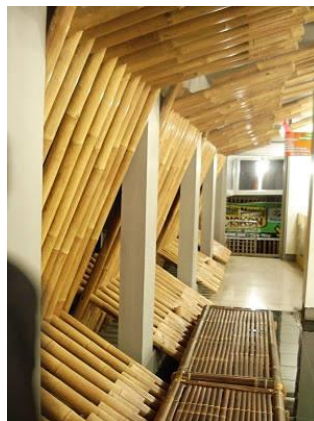
Figure 5. Windows finishing, so that the function remains optimal, the window grille opened with bamboo material
