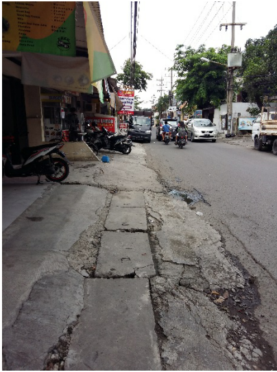
Fig. 3 The accessible pathway were found nearby the PCU Main Campus, only there was no curb ramps and no stable, firm, and slip-resistant walking surfaces. Therefore the non PwDs could access but PwDs would find difficulty.
