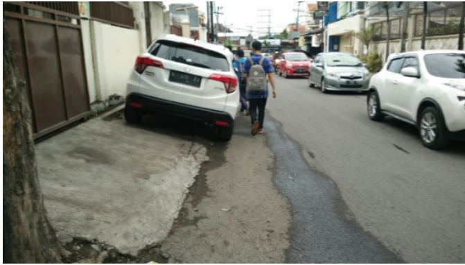
Fig. 7 The sidewalk which cross slopes exceeded 1:50 causing more danger for pedestrian using crutch, walking stick or wheelchair.
