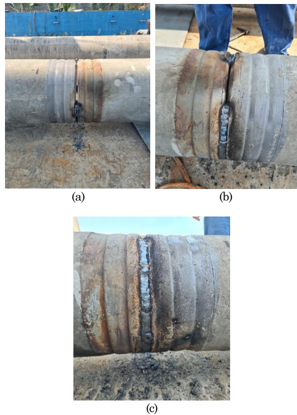
Figure 7. (a) Welding at Four Points; (b) Welding at Half Circle; (c) Welding Full Circle
