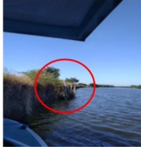
Figure 2. Damaged Retaining Wall
