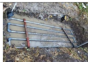
Figure 4. The bottom pipe is at 100 cm depth.
