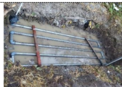
Figure 4. The bottom pipe is at 100 cm depth.
