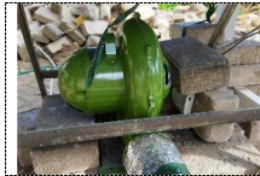
Figure 3. The blower, that blows fresh air into pipe.
