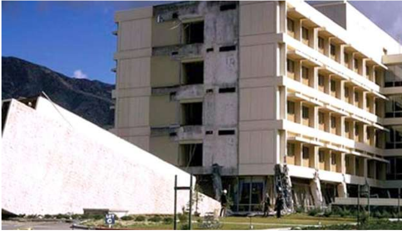
Gambar 29b. Olive View Hospital Pounding dng Core, San Fernando, California, Tower Tangga Wing A, B, D Runtuh Karena Pounding https://quake06.stanford.edu/centennial/tour/images/10-06-IMG0036.jpg , diunduh Mei 2019
