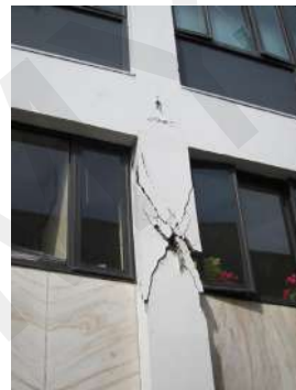
Gambar 44. Kegagalan Short Column
