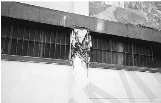
Gambar 43. Kegagalan Short Column
