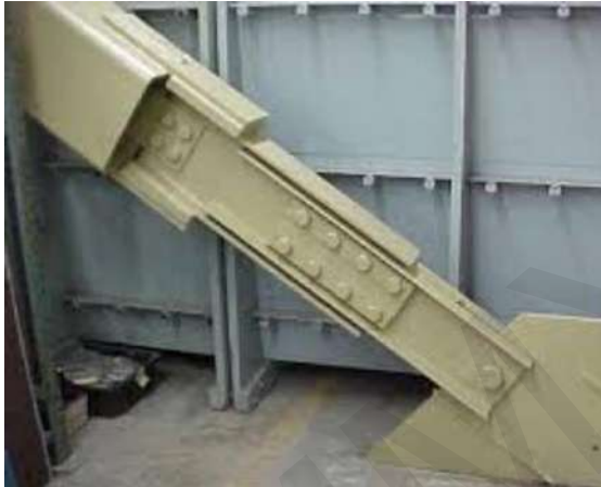
Gambar 101. “Pall” Friction Slotted-Bolted Damper Terpasang di Truss Baja https://www.iitk.ac.in/nicee/wcee/article/13_1955.pdf , diunduh Juni 2022
