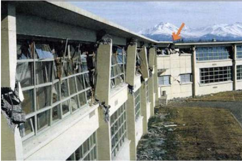
Gambar 19e. Kegagalan Struktur West Anchorage High Shool
