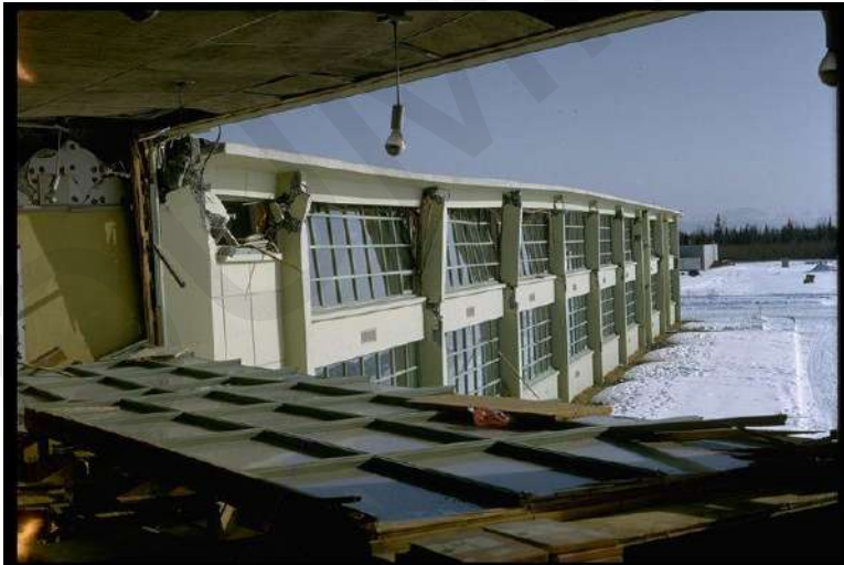
Gambar 19f. Kegagalan Struktur West Anchorage High Shool
