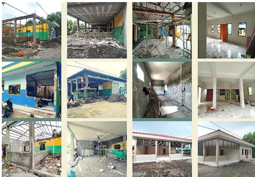
Figure 13. The construction process of the Kampung Herbal Jangkungan Nginden Surabaya Library building was carried out by community members with the supervision of students and lecturers (Photo: Nathania, 2021).
