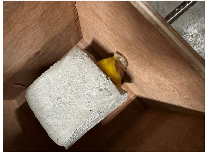
Figure 6. Protection for the Steel Reinforcement using Combination of Clear Tape, PVC Pipe (covered), and Clay
