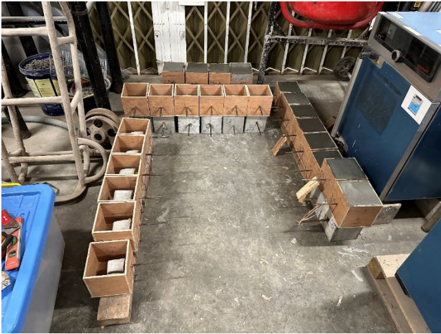
Figure 5. Small Cubes Placed in the Formwork (left) and Grouting Material used as Filler (right)
