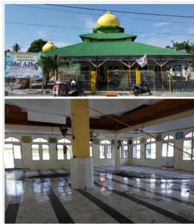
Figure 5. Nurulhasanah Pengawu Mosque condition after earthquake
