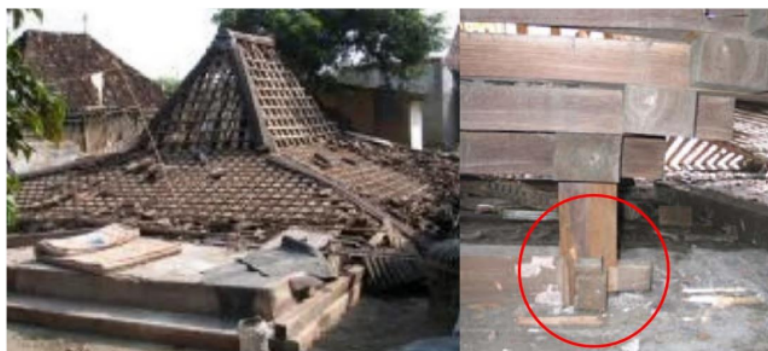
Fig. 3: Joglo which completely collapsed due to the 2006 earthquake; the four main pillars ( saka guru ) in the core structure ( rong-rongan ) were broken.
