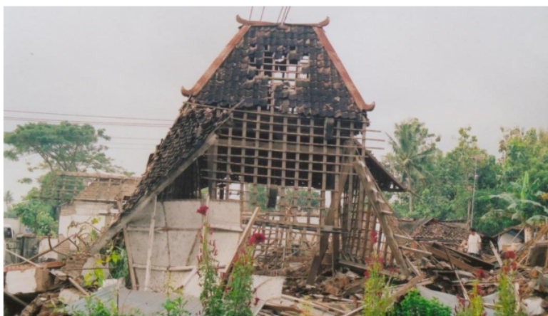
Fig. 2: A heavy damage joglo due to the 2006 earthquake: it but did not collapse completely; the core structure ( rong-rongan ) remains.
