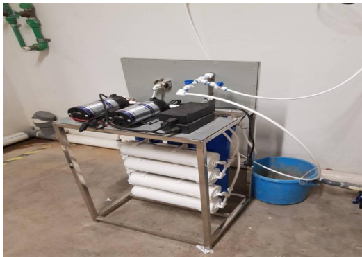
(c) Reverse Osmosis
