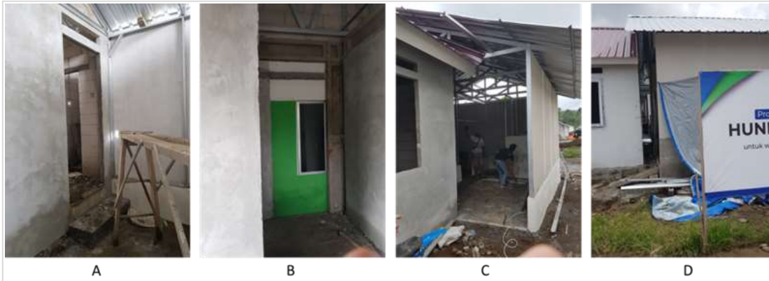
Figure 13. Problems in integration of the two housings
