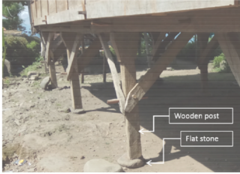
Fig. 6 The foundation structure of stilt house: a wooden post placed on a flat stone
